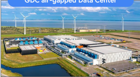
GDC air-gapped Data Center
